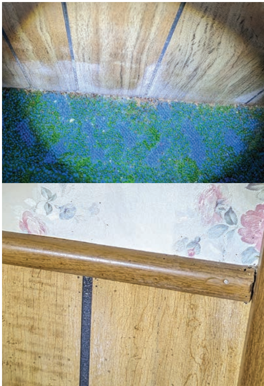
Figure 3 Evidence of long-term and structural infestation.
