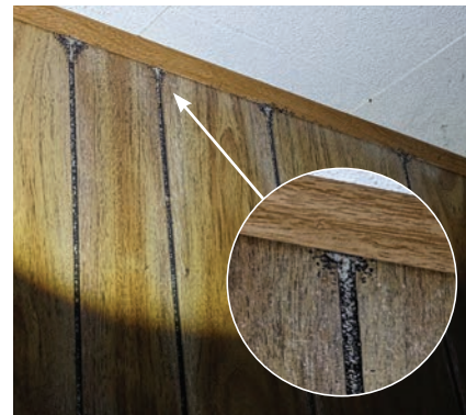
Figure 2 The infestation had spread to the ceiling mouldings.
