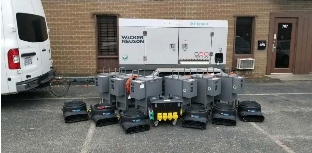
Figure 1: Bug Bakers™ generator and heating equipment
